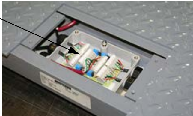
Figure 2-4. Junction Box Opened
