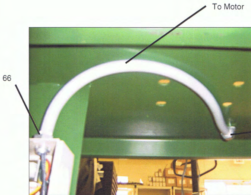
ELECTRICAL WIRE TO MOTOR
