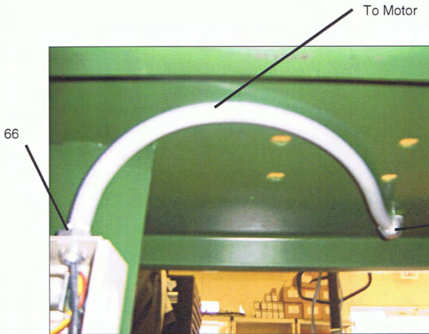
ELECTRICAL WIRE TO MOTOR
