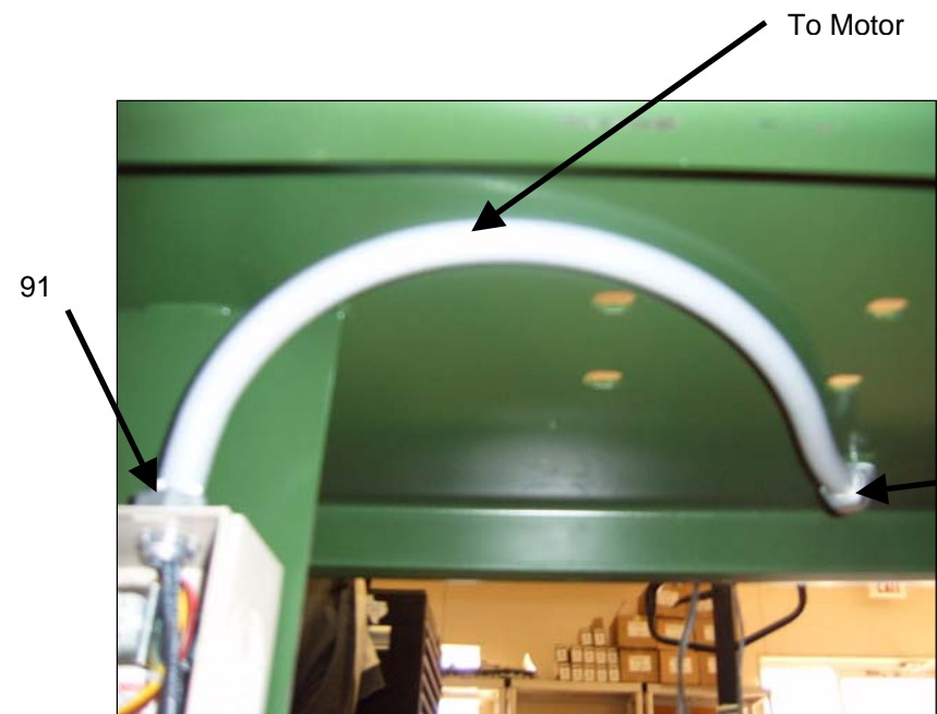
ELECTRICAL WIRE TO MOTOR
